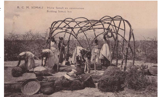
Building a traditional Somali collapsible house of "Aqal". The hoops are often made from the roots of Acacia bussei .
